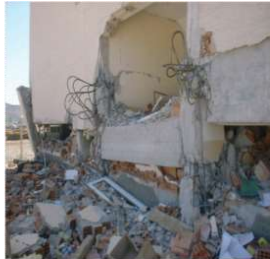
Fig. 1. Failure of column with eccentric connection
